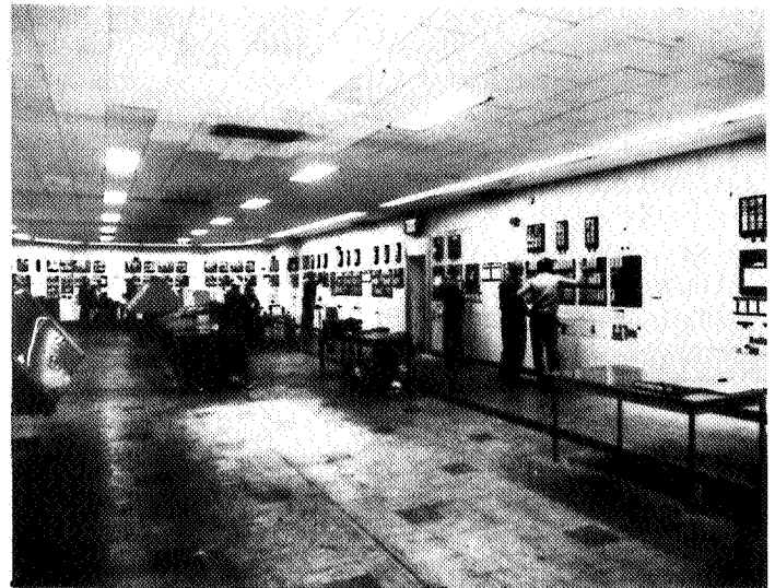
Figure 4. Ammonia plant central control room.
